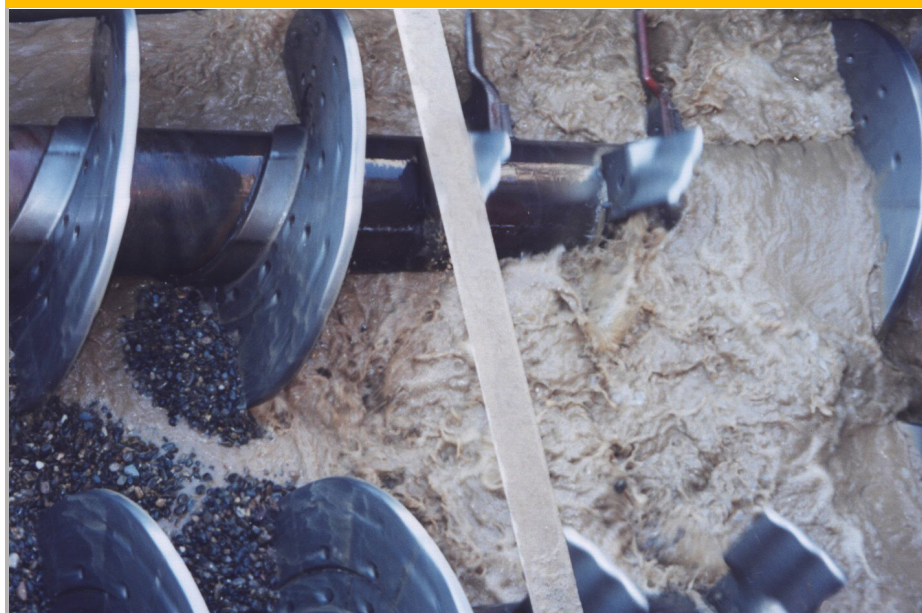
A look inside at the paddles and shaft of a coarse material screw washer.
